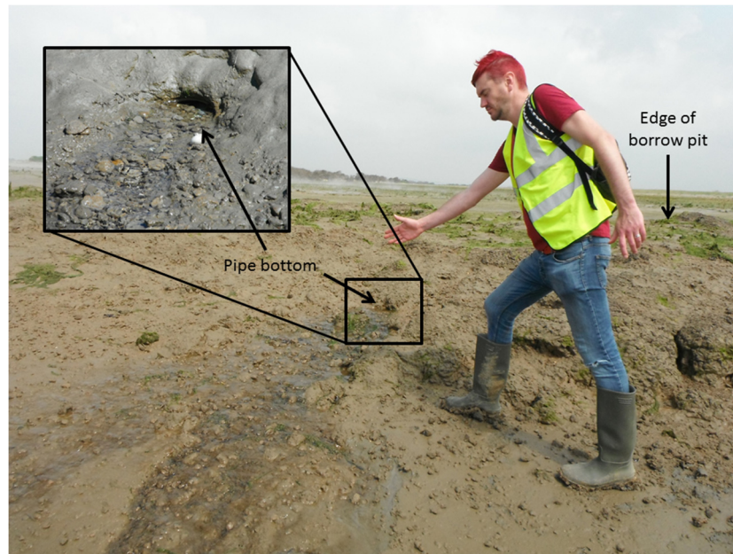
Fig. 7. Water flowing from the bottom of a pipe (inset) through the bank of the borrow pit in June 2014.
