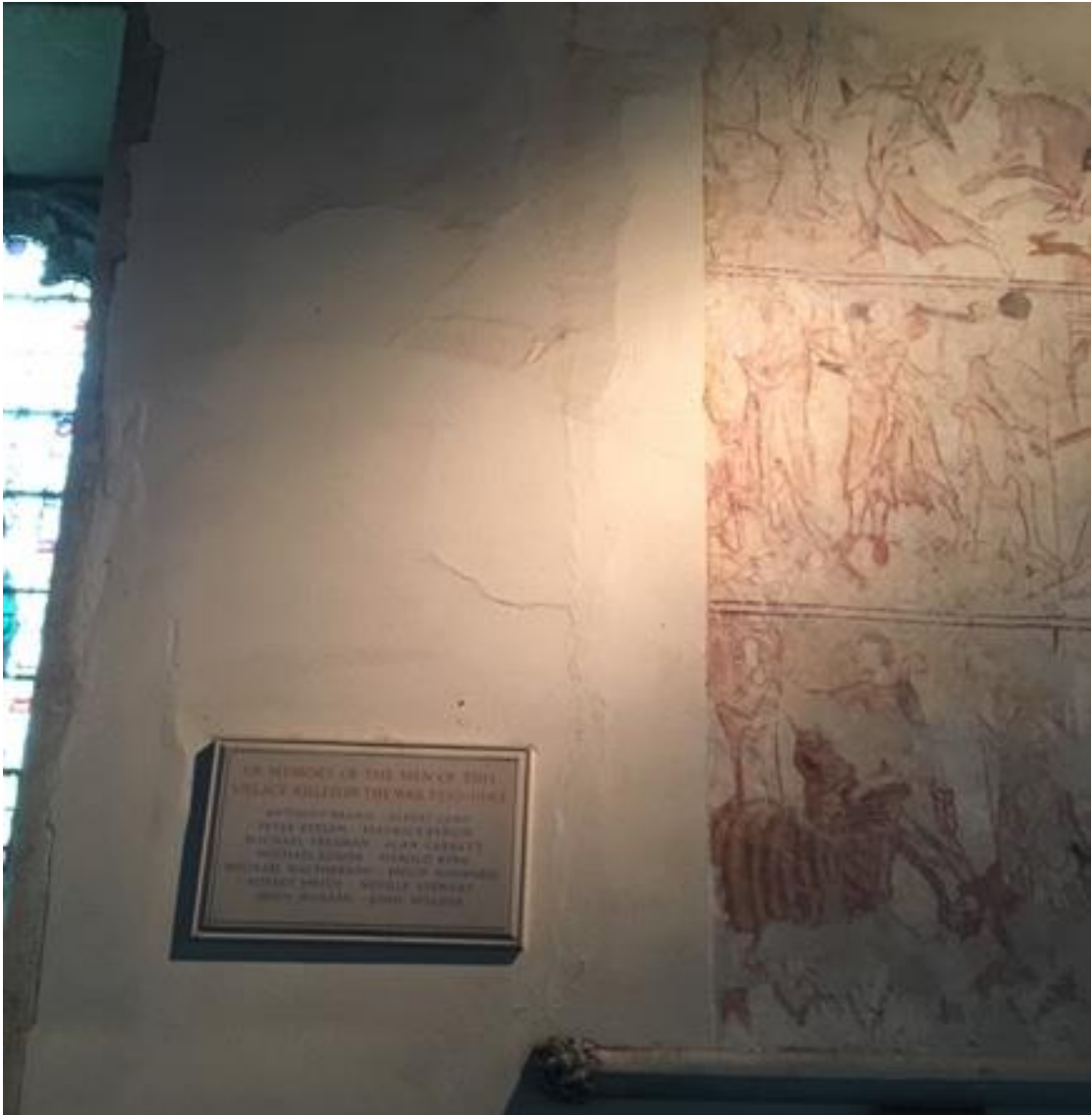
Figure 3.6: St Nicholas, Charlwood, Surrey. St Margaret Cycle (14thC). Showing damage to the left-hand side of the paintings.
