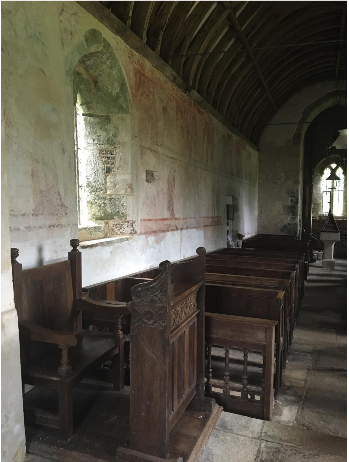
Figure 1.9a: St Mary the Virgin, Tarrant Crawford, Dorset. South wall of the nave looking west. Overview of the 13th-14thC wall paintings of the St Margaret Cycle (upper tier of paintings).
