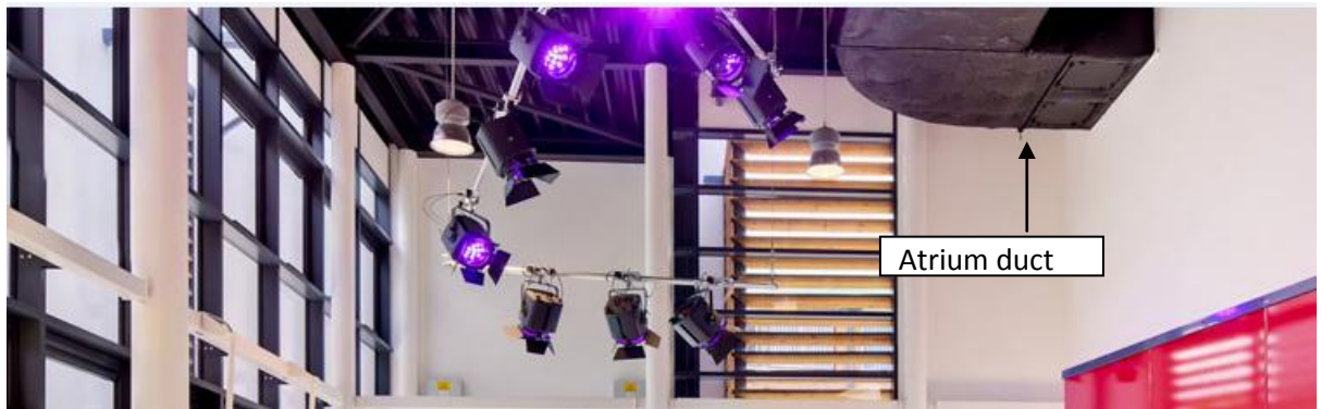
Figure 7-5 Exposed atrium duct (details from the architects' image of the complete building)
