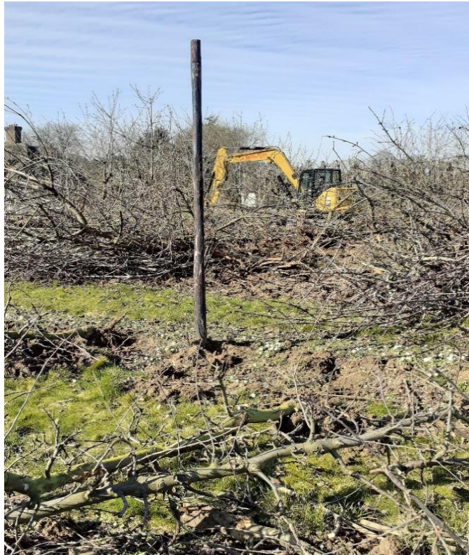
Fig 6.1. Grubbing of a nine-year-old apple orchard on the 14 th of March 2022, which had a mixture of Rubens and Gala trees grown on M9 rootstocks at NIAB East Malling. Image taken by Catherine Chapman on 15 th March 2022.
