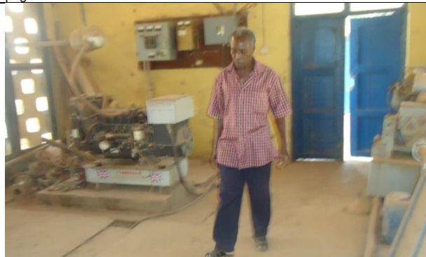
Genset in Daffiama. A similar one is in Gwollu
