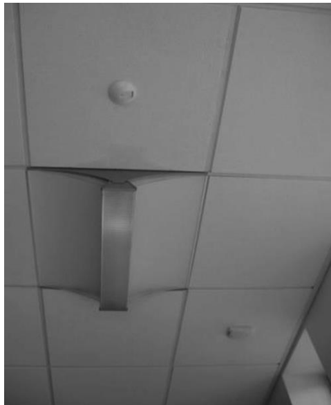
Figure 6. Lighting and PIR sensors.
