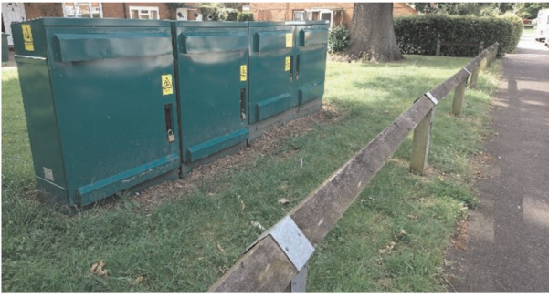
Fig. 1 ESMU with one PEU (on the right) and two ESUs (on the left) installed on a grass verge near a footpath in residential area in Bracknell, UK
