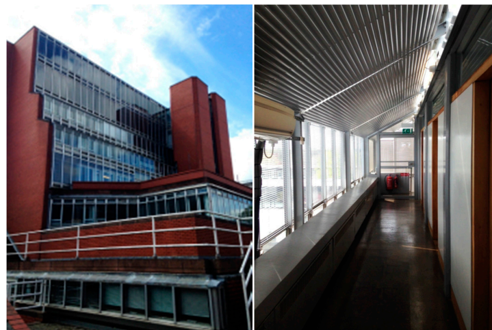
Figure 6. Excessive glazing and solar heat gain contribute to overheating.
