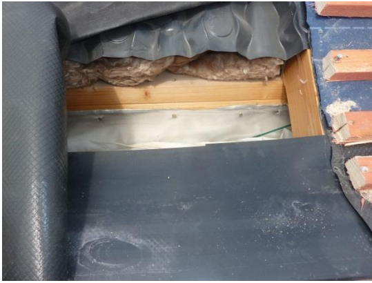
Figure 4.27: Ventilation gap closed. Batten has trapped felt and rafter tray has been compressed against the felt by the insulation, thus blocking off the air path
