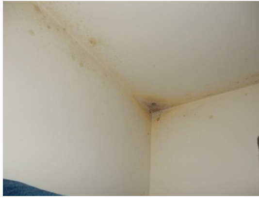
Figure 4.28: Mould growth to wall/ceiling junction 1
