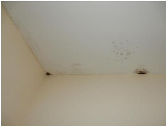
Figure 4.29: Mould growth at wall/ceiling junction 2
