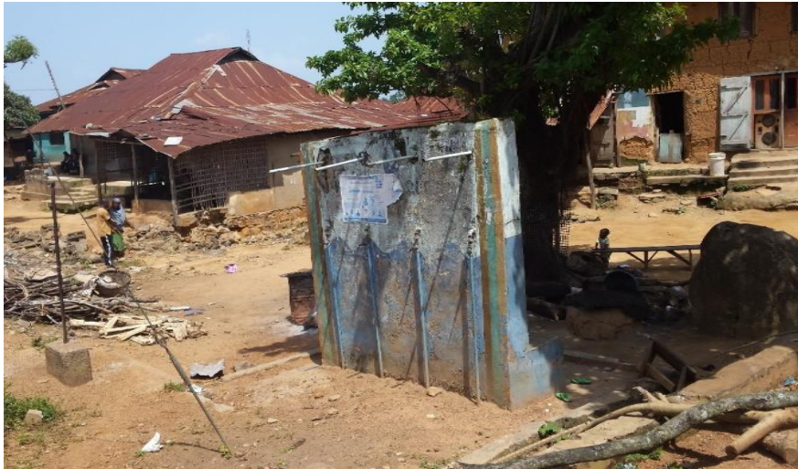
Figure 4.7: Non-functional borehole in Igogo Idoka
