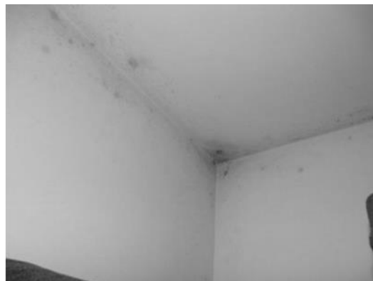
(b) The air path blocked off, resulting in mould growth
