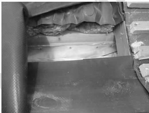
(a) Batten has trapped felt and rafter tray has been compressed against the felt by the insulation
