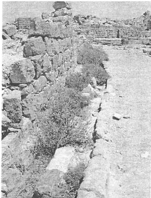
Fig. 6. Water-collecting channel. Note vegetation growing in channel, indicating that it still serves as a conduit for water.
