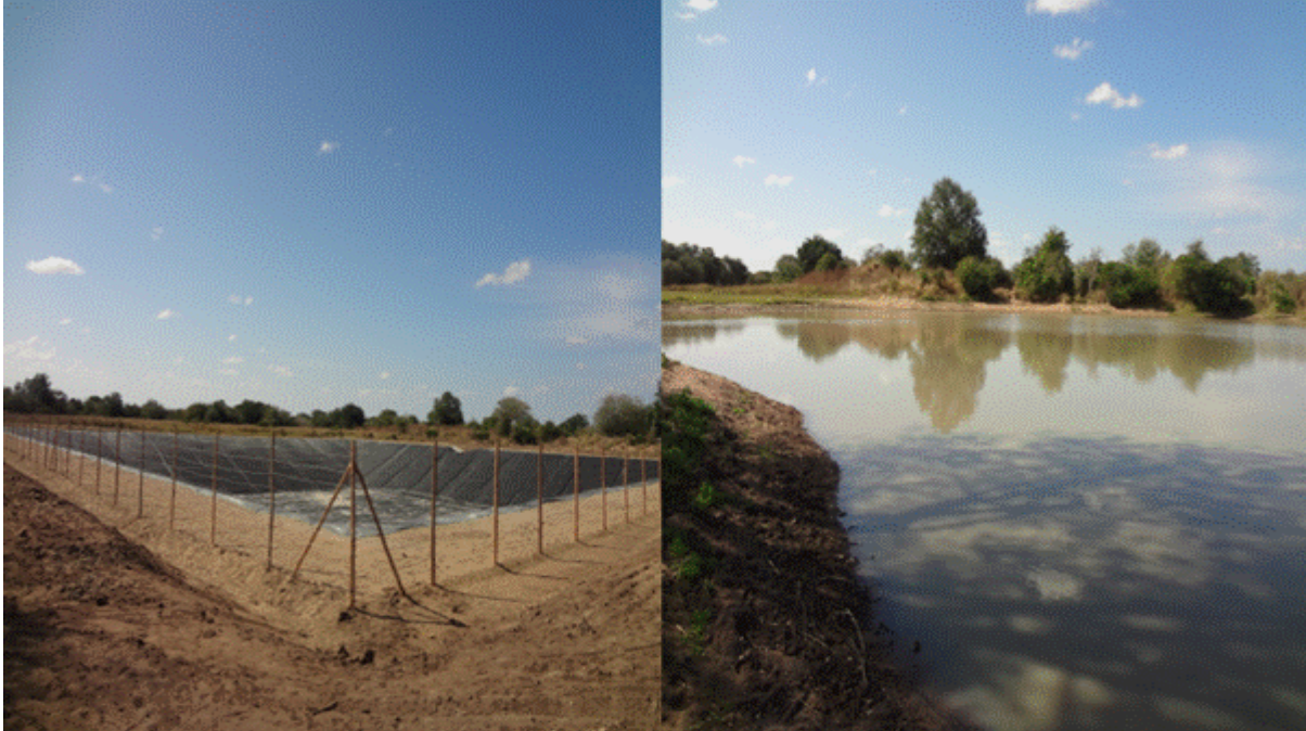
Water reservoir under construction (left) and the source of water to the reservoir (right) in Mbala-Vala, Guija (source: Author, July 2017)
